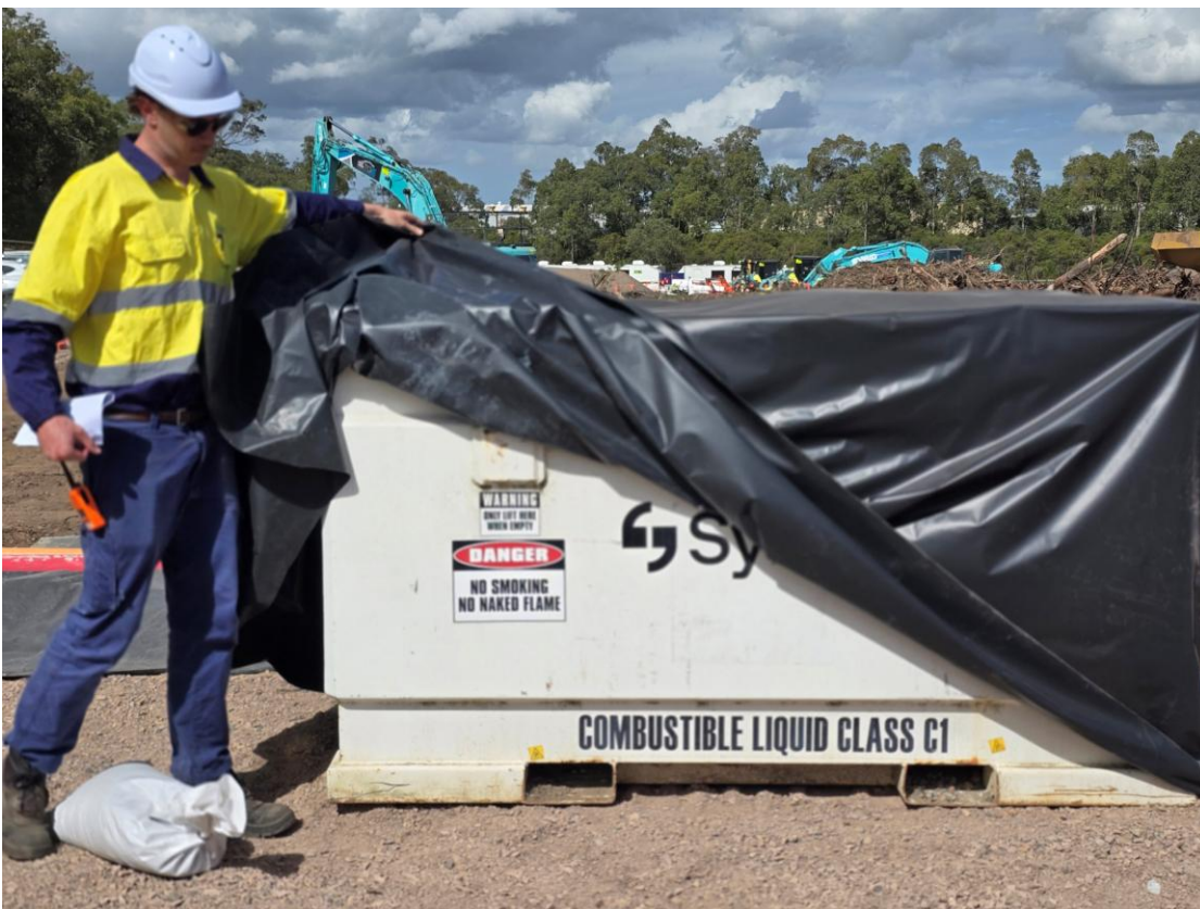
Plate 28 – Self-bunded diesel tank in refuelling area
