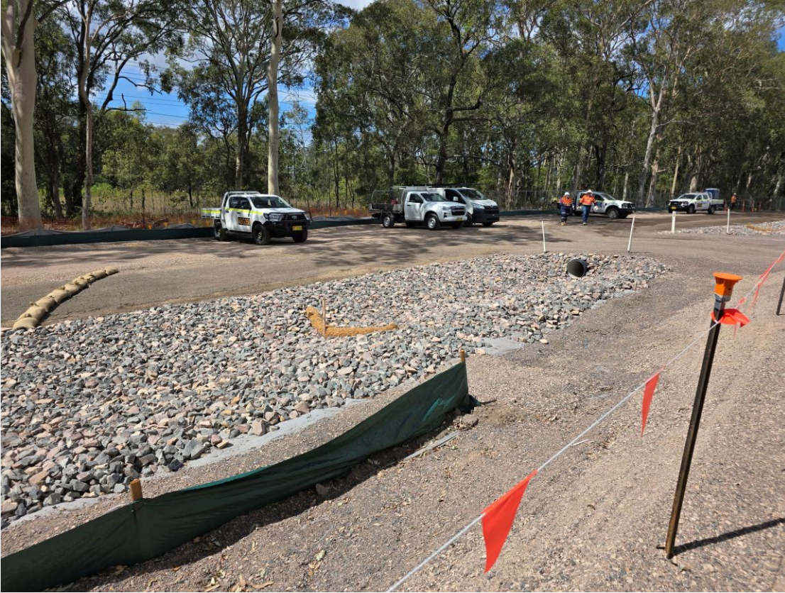
Plate 23 – Rock drains along internal access road
