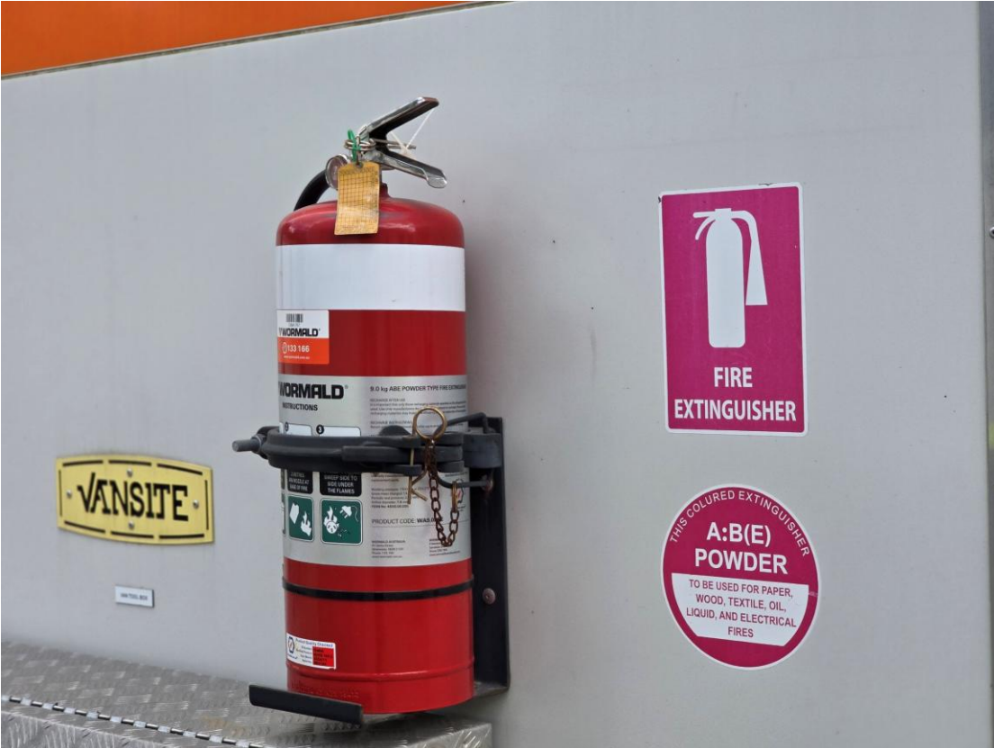
Plate 32 – Portable fire extinguisher
