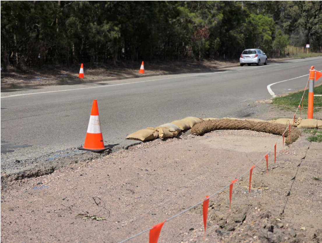
Plate 7 – Erosion and sediment controls at the access point off Old Punt Road #2
