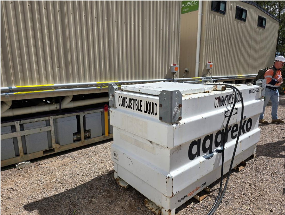
Plate 27 – Self-bunded diesel tank for generator at site offices
