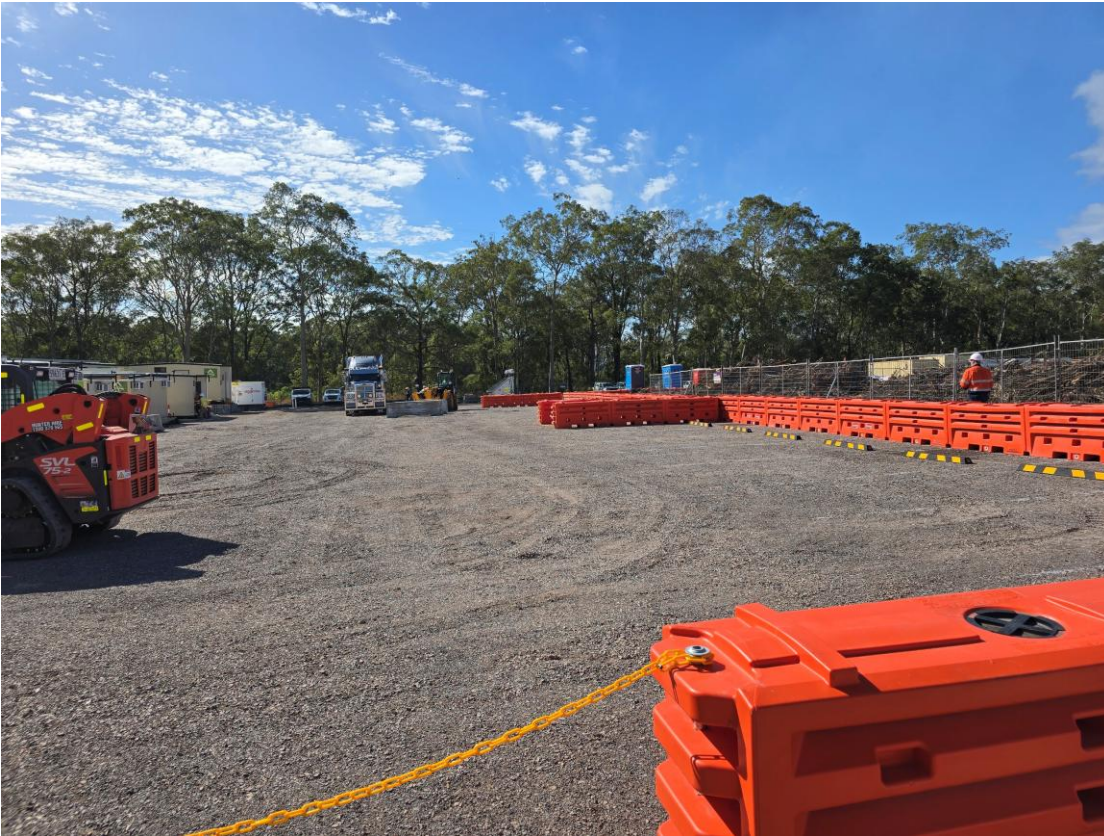
Plate 11 – Carpark and unloading area (site offices were being installed at the time of audit)
