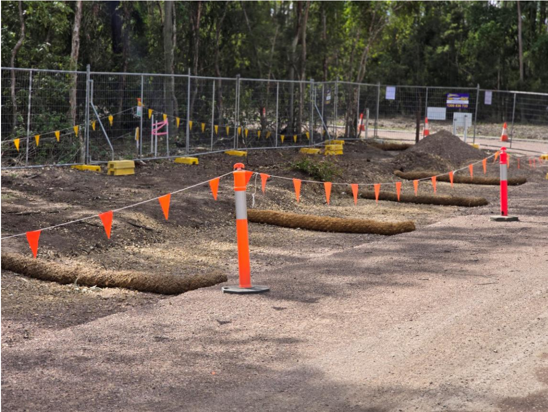
Plate 6 – Erosion and sediment controls at the access point off Old Punt Road #1
