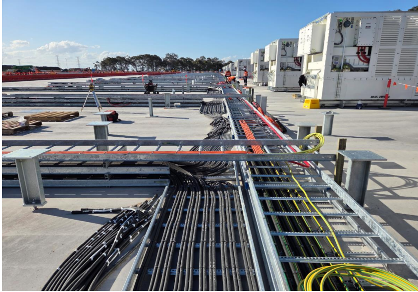
Cable reticulation and RMU's on BESS combislab
