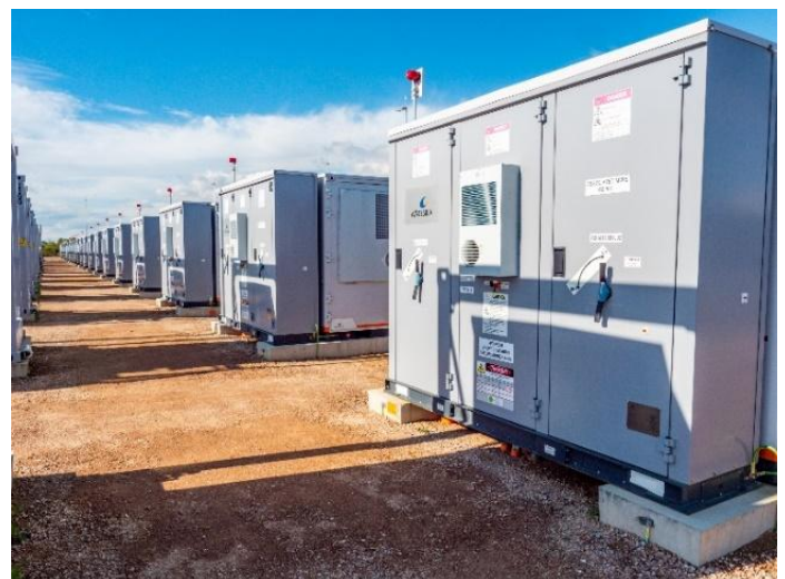
Image: AGL's 250 MW grid-scale battery at Torrens Island South Australia
