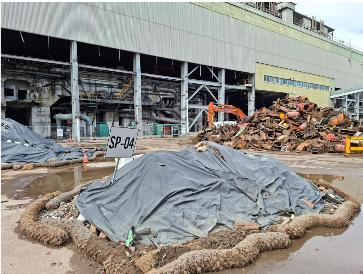
Plate 4 – Waste stockpiles & signage in the Liddell demolition area
