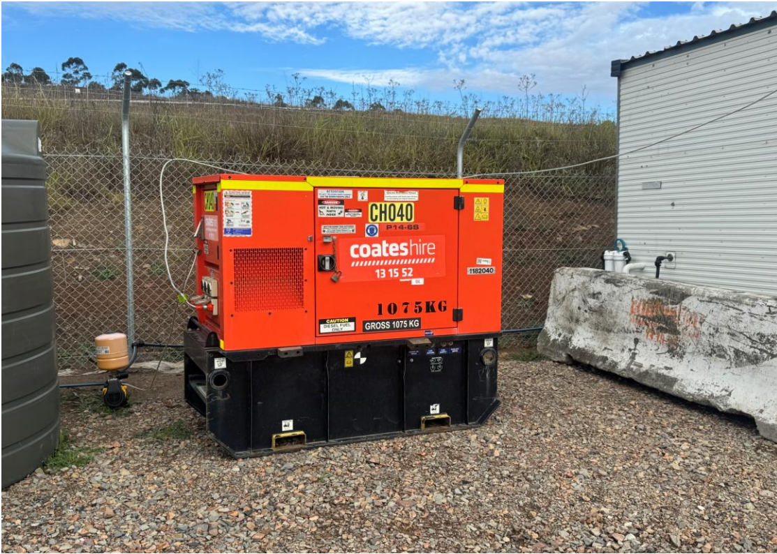
Plate 13 – Bunded diesel generator outside the asbestos disposal facility
