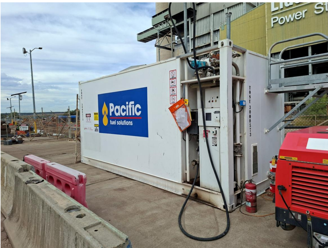
Plate 12 – Self-bunded diesel storage tank at the Liddell demolition area
