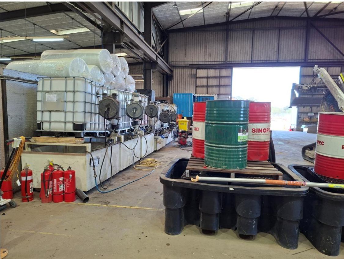
Plate 16 – Bunded chemicals and fire fighting equipment in store area of Liddell Power Station
