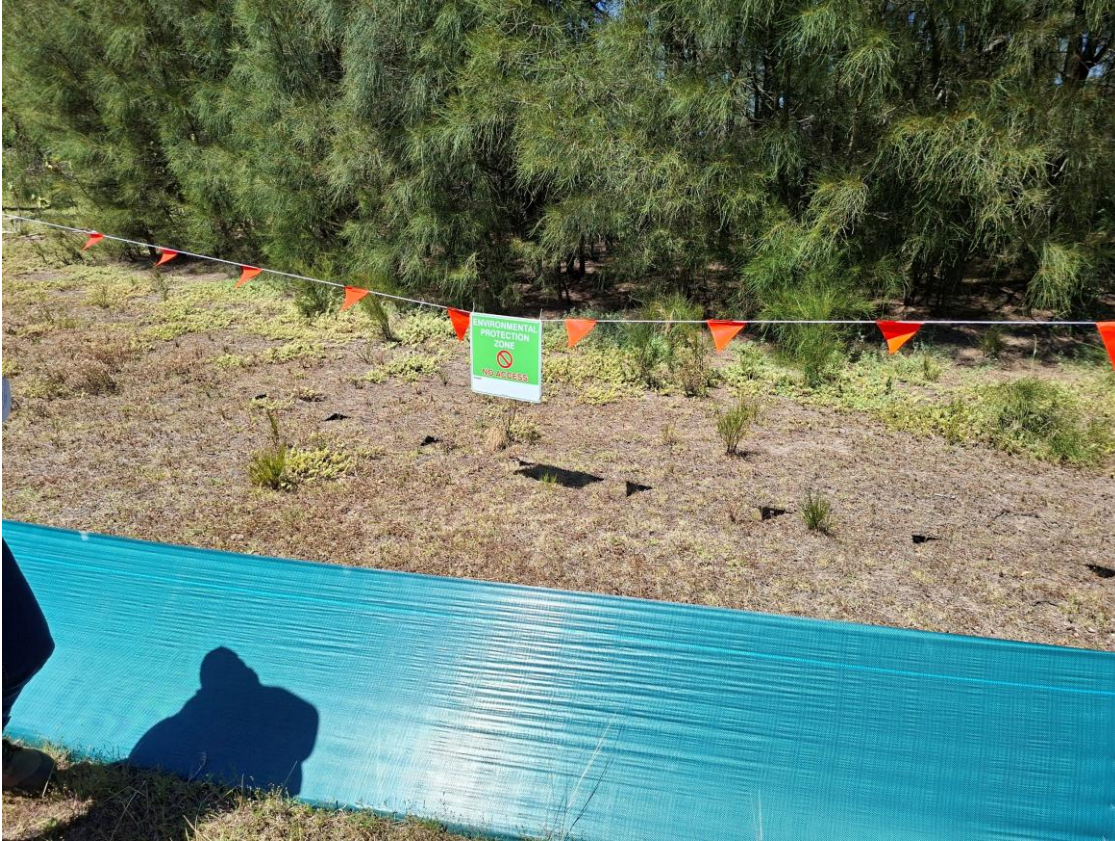
Plate 29 – Frog exclusion fencing and 'No Go' zones demarcated at Liddell Power Station oil and grit trap works area
