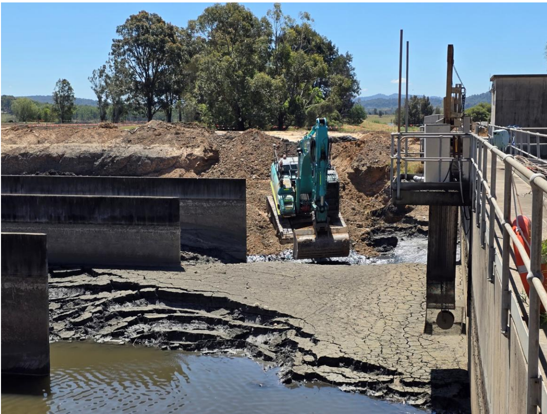
Plate 2 - Excavator desilting the Liddell oil and grit trap within Stage 1 works area
