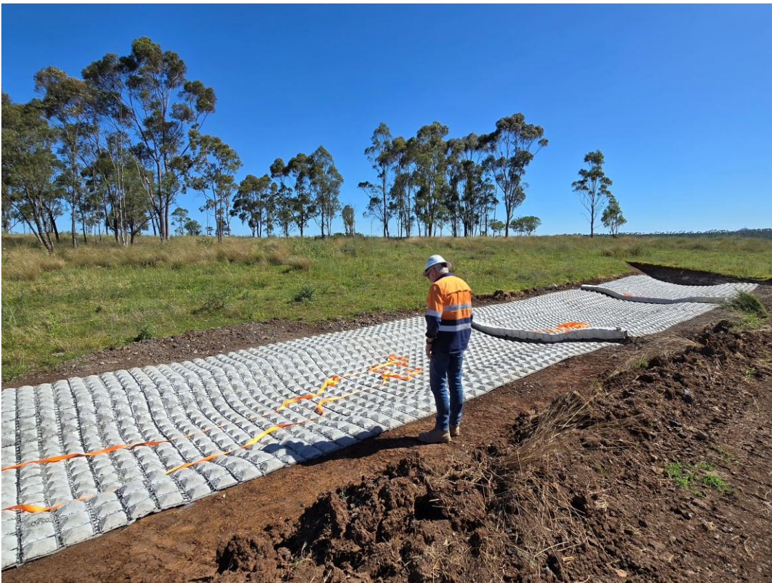
Plate 12 – Geofabric lining for drains to exclude clean water from asbestos disposal facility
