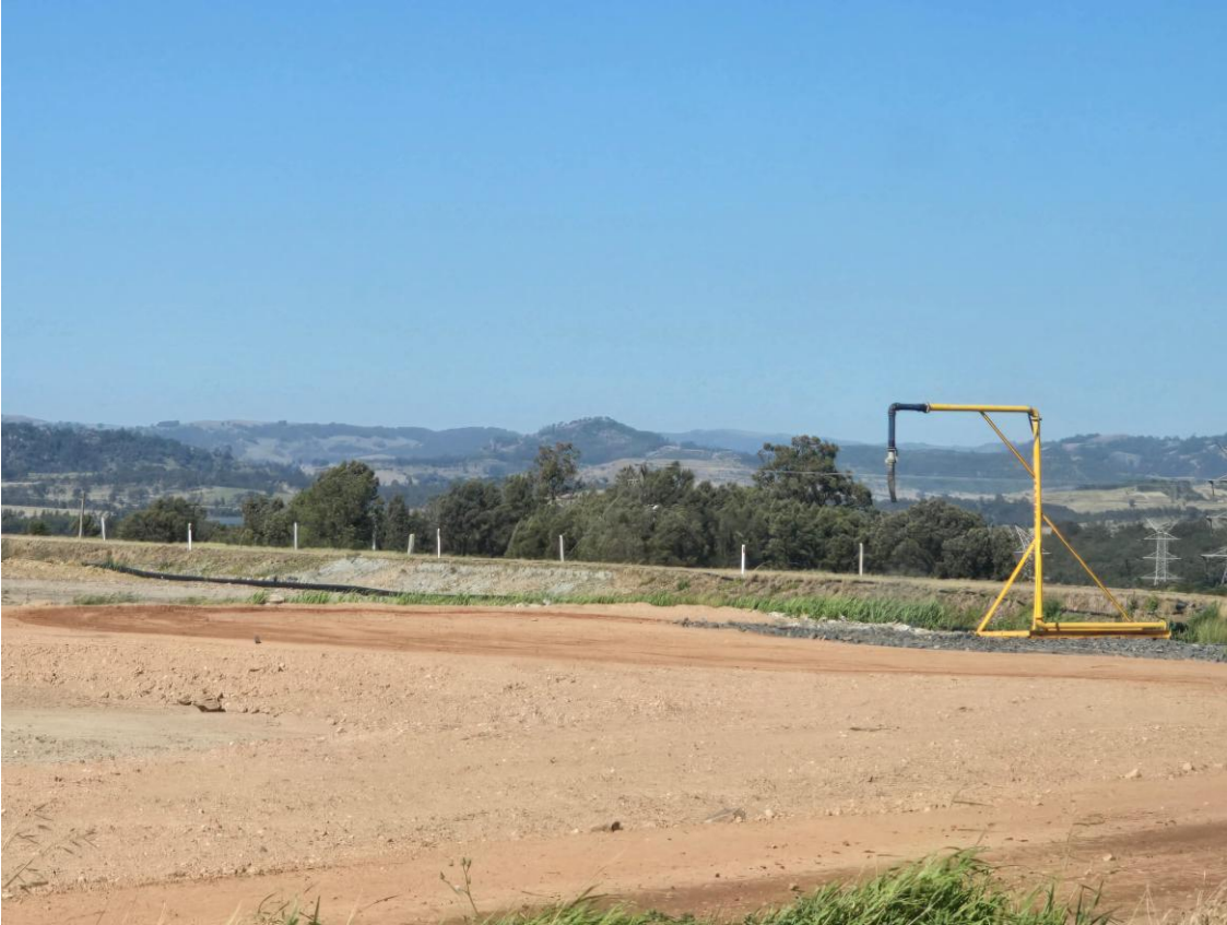
Plate 7 – Fill point in place on the haul road to the asbestos disposal facility construction
