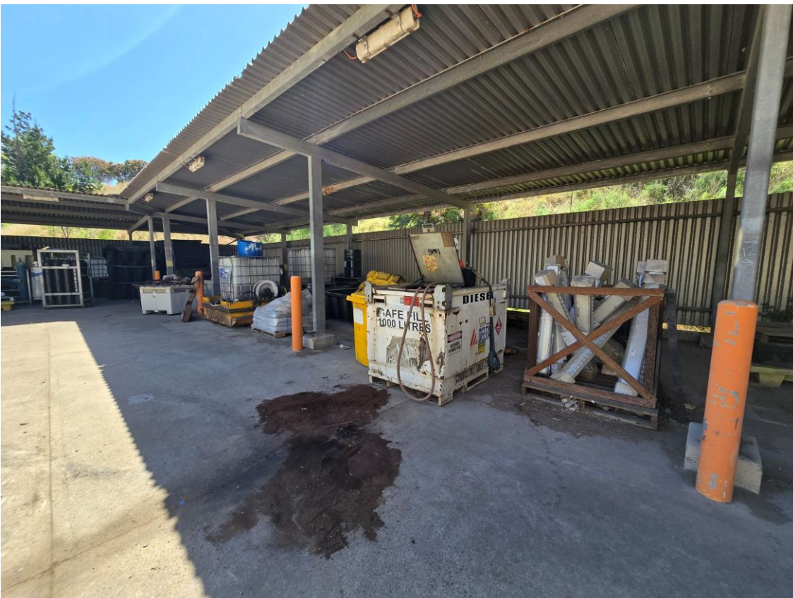
Plate 22 – Diesel spill at 1,000 L diesel storage tank
