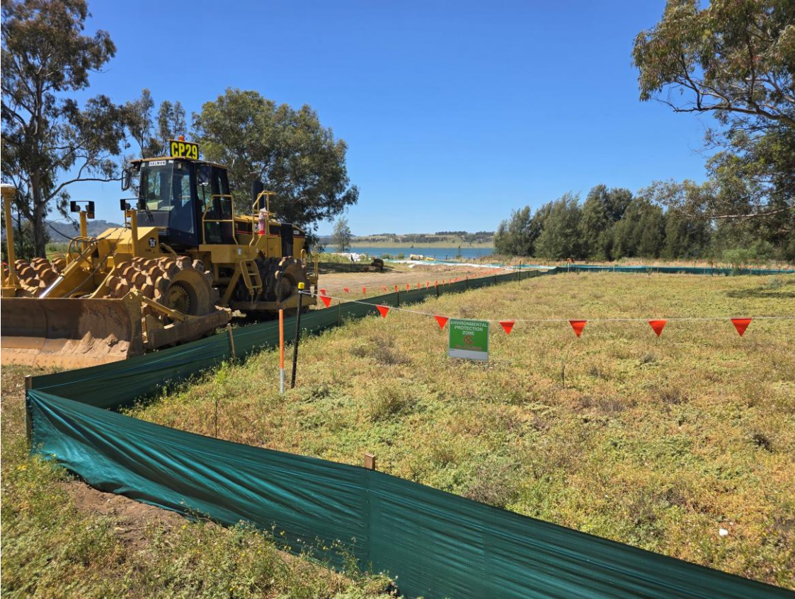
Plate 13 – Erosion and sediment controls installed for oil and grit trap basin enlargement
