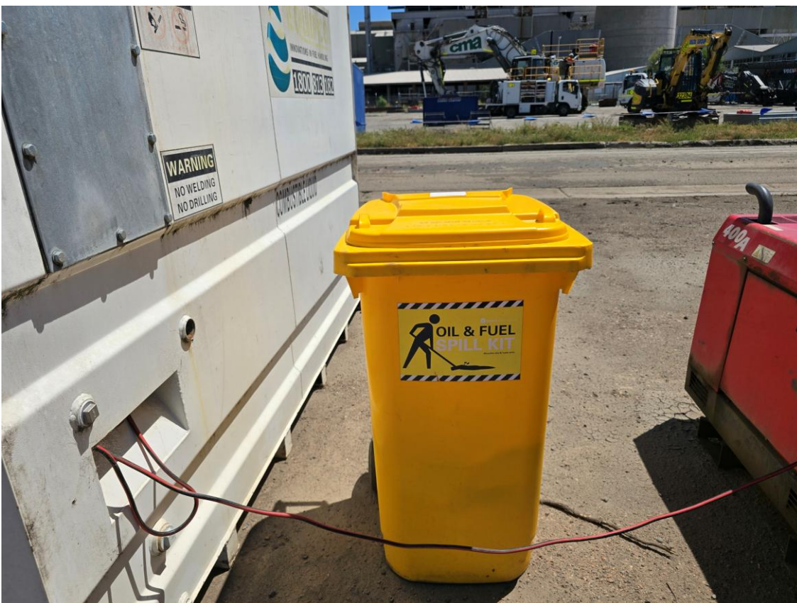
Plate 18 – Spill kit next to fuel storage tank
