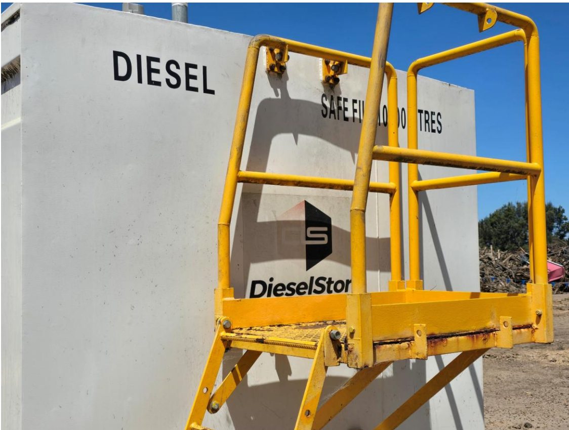
Plate 20 – 10,000 L Self bunded diesel storage tank
