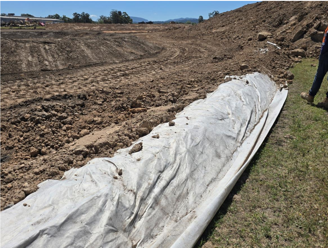
Plate 14 – Bund plastic lining to prevent erosion
