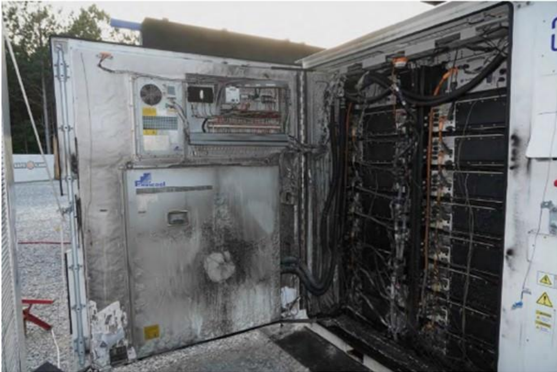
Plate 8: Inside the Initiating Unit after the BBDT
