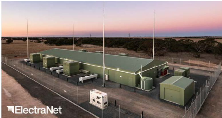
Dalrymple North Battery Energy Storage System
